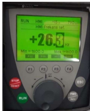
Figure 4.19. Frequency inverter (Schneider electric, Altivar 71, 4 kW)
